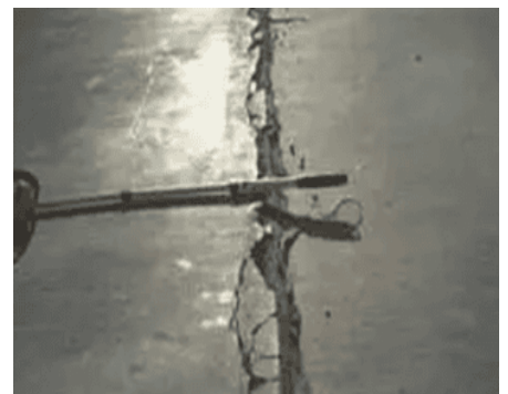
Image: Jointed Concrete Pavement in Poor Condition by Faulting Metric
