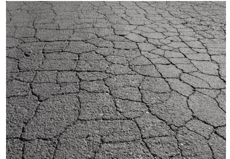
Image: Asphalt Pavement in Poor Condition by Cracking Metric (Source: Sable Asphalt)
