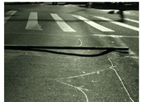
Image: Asphalt Pavement in Poor Condition by Rutting Metric (Source: G.H. Shafabakhsh (2014))
